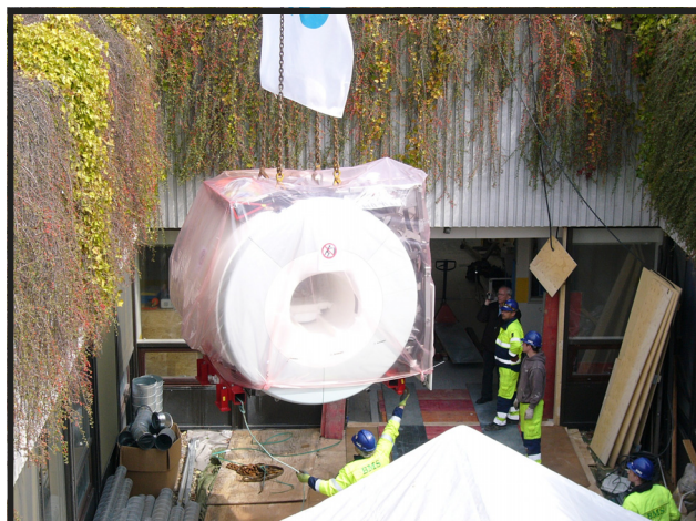
The magnet of one of the new MR scanners being lowered into the hospital building in March 2010.
